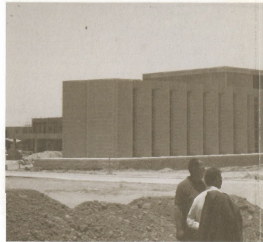
Section of new King Faisal Specialist Hospital rises in Riyadh, Arabia. The hospital will make extensive use of HP medical equipment.
